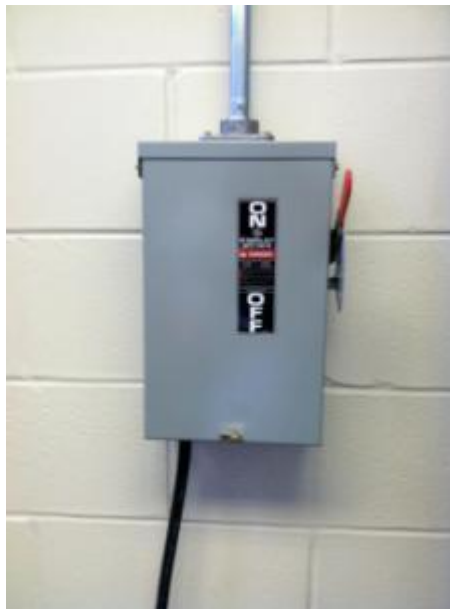
Figure C.1 Main power source switch.
