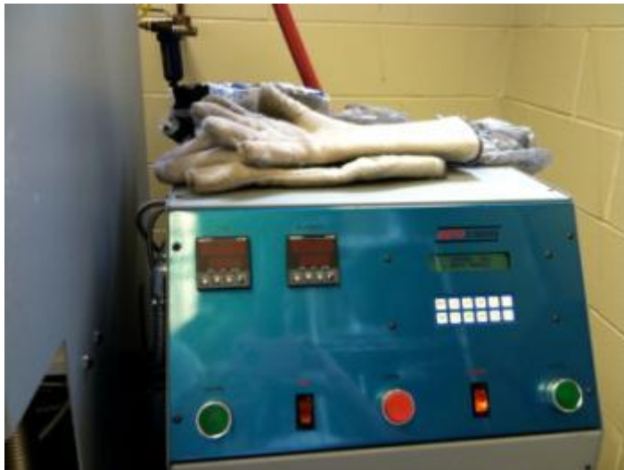
Figure C.3 Instrument control panel.
